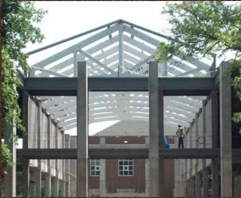
S.W.S. fabricated wood trusses for the Wallace Dining Hall, shown here while still under construction.
