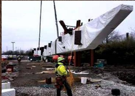
The erection crew worked carefully installing the massive beams. The above photo gives you an idea of just how large the beams are.
